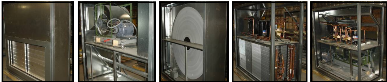
From left: The end section contains the OA damper; the next section contains the exhaust blower (top) and OA filter rack (bottom); the middle section houses the heat wheel; the next section contains the DX and Hot Gas Reheat coils (bottom) and two compressors (top); and the last section houses the twin supply blowers (bottom) and another two compressors (top).
