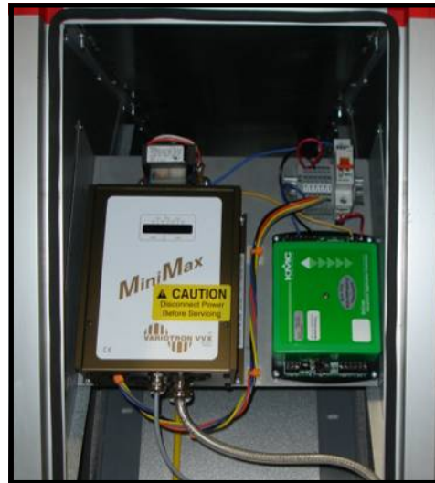
Xetex DDC controller (right) alongside MiniMax multifunction heat wheel VFD (left)
