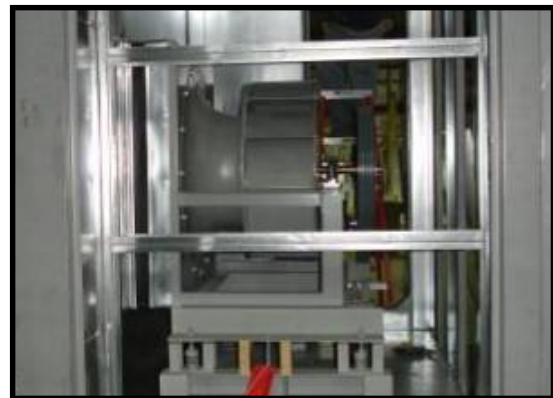
Air foil plenum blower section.
