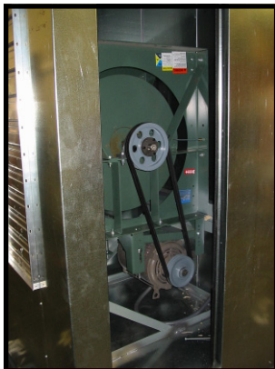
15hp Exhaust Air Blower
