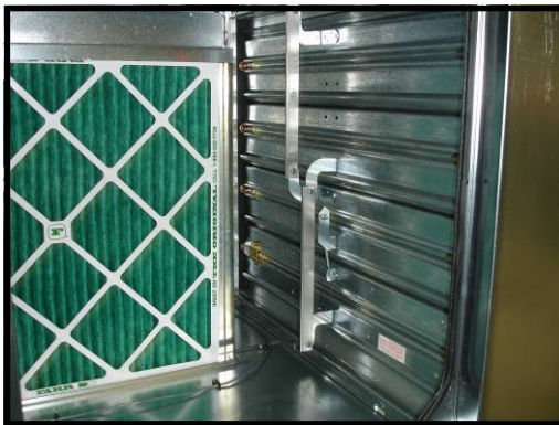
OA Damper and Filters
