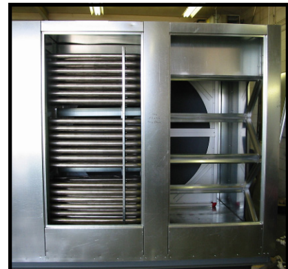
Supply Air (on left w/gas fired furnace) and Return Air (on right) through the heat wheel
