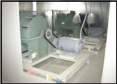
Dual blower and motor configuration
