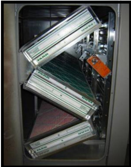
Filter and Damper Access
