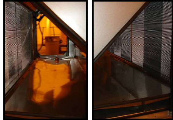
DX Coil for cooling and dehumidification (right), Hot Gas Bypass coil for Reheat (left)
