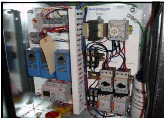
Controls: motor starters, fuses/breakers, transformer, service switch, and terminal points
