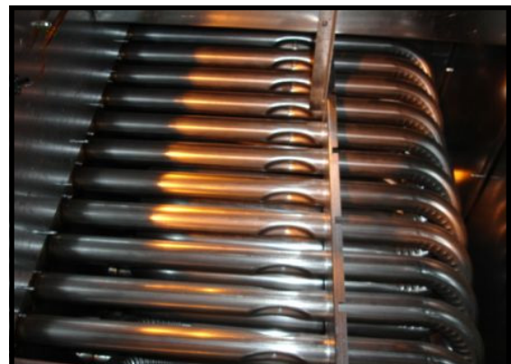
The IAQ line accommodates many options. This unit has an indirect gas fired heater.
