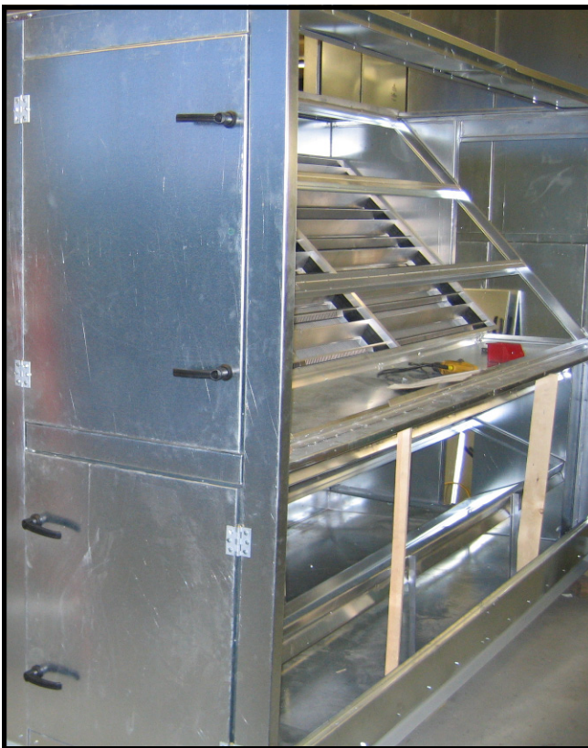
With End Panels Removed, the Face-and-Bypass Damper behind the Filter Rack is visible.
