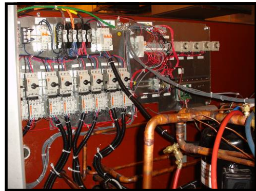
Controls for a DX compressor system including Compressor Motor Contactors and Starters and Timed Relays
